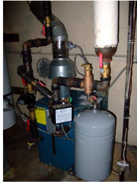
Figure 6b. Typical boiler found in recently renovated Broadmoor development.
