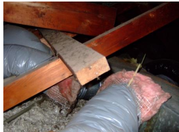
Figure 15b. Disconnected flex supply duct
