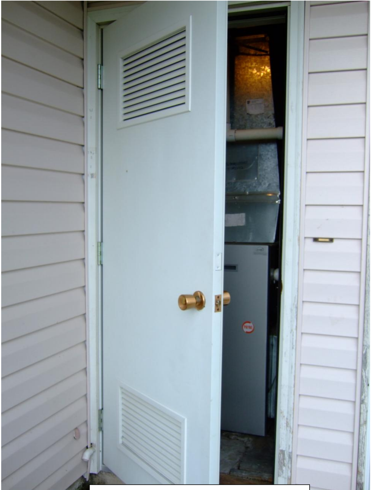
Exterior access unconditioned mechanical closet typical in Davis Hill and New Hillside developments
