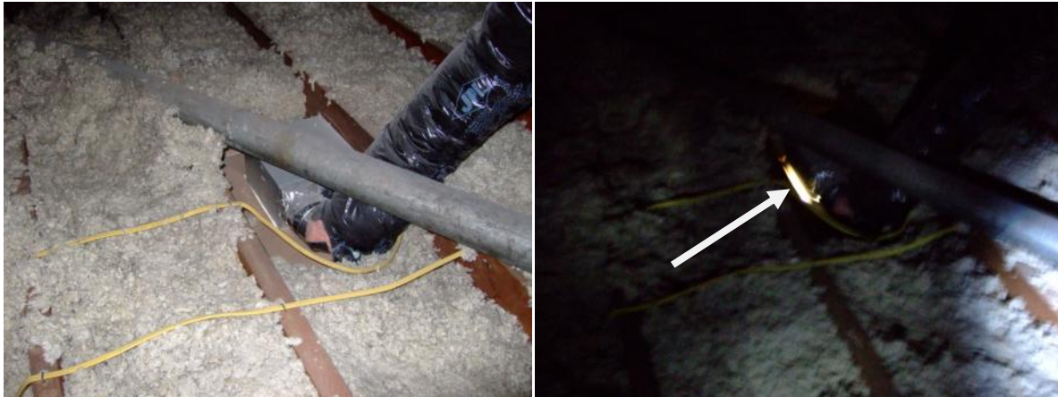
Figure 10. Bathroom exhaust fan installation showing significantly compromised air and thermal barrier
