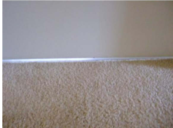
Insufficient return area at door undercut causing pressurization of bedrooms
