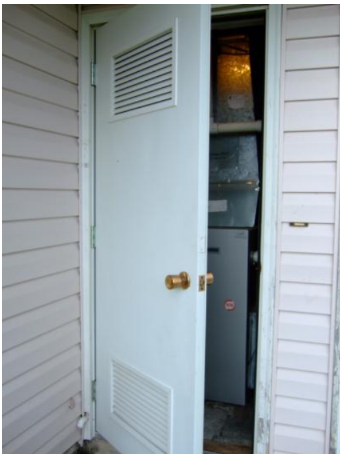
Figure 8a. Typical mechanical closet in Davis Hill and New Hillside developments.
