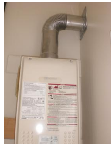
Figure 7c. Typical 0.82 EF natural gas tankless water heater found in Miller Hill homes
