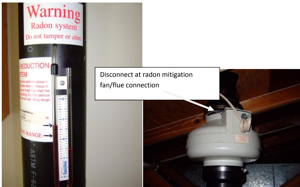
Figure 16. Radon mitigation system, Beachwood development
