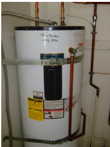
Figure 7a. Typical 0.90+ EF electric tank water heater
