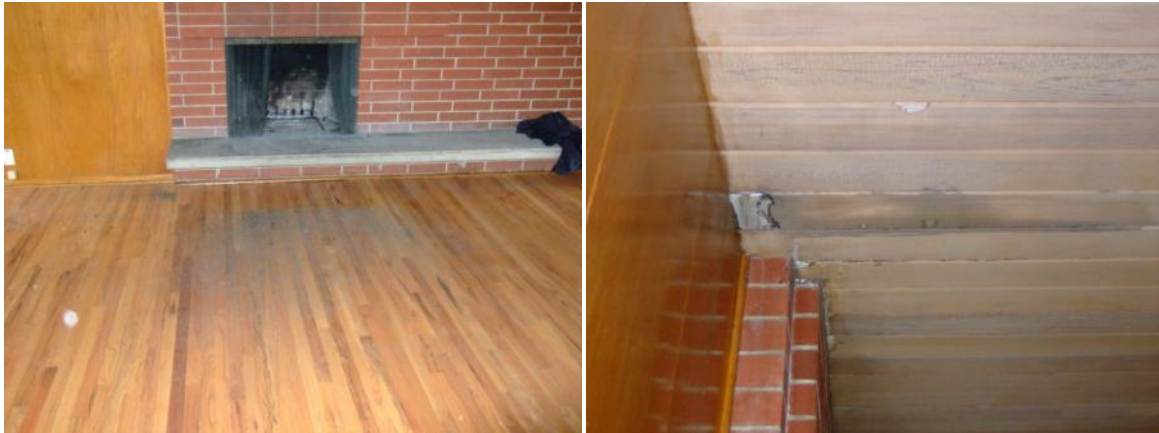
Fireplace flue without doors and penetration are significant air leaks
