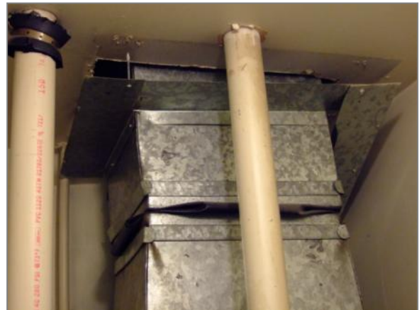
Figure 14b. Typical air barrier deficiencies
