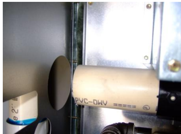
Figure 8b. Combustion supply air intake cut at furnace cabinet.
