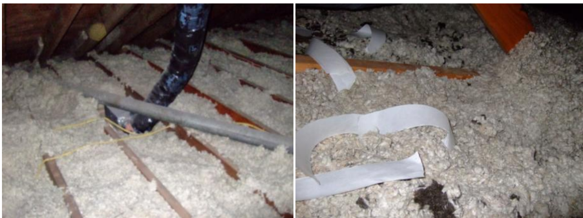
Figure 9. Attic insulation in two different plan types showing compressed and inconsistent fill
