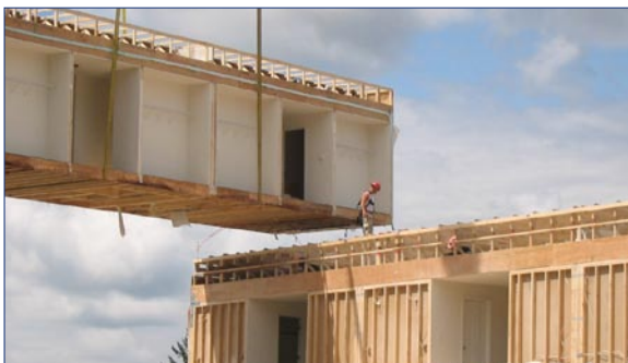
Figure 2. The Ft. Lewis project is the first military housing project to use modular construction. With modular construction energy efficiency can be implemented cost effectively on a large scale.
