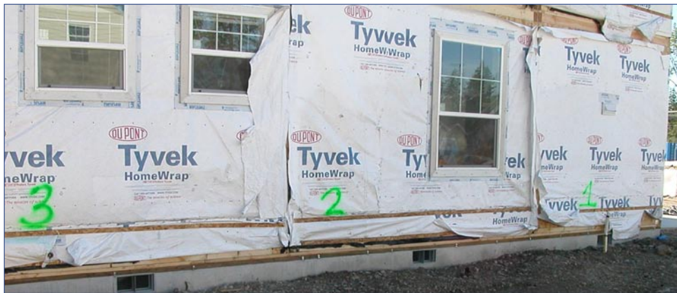
Figure 4. Modules are numbered for placement. Housewrap and window flashing has been carefully applied at the factory to exterior walls. Housewrap flaps are provided for overlap with surrounding modules. The housewrap is overlapped shingle-style to create a drainage plain beneath exterior cladding. The foundation wall for the crawlspace can be seen at the base of the walls.
