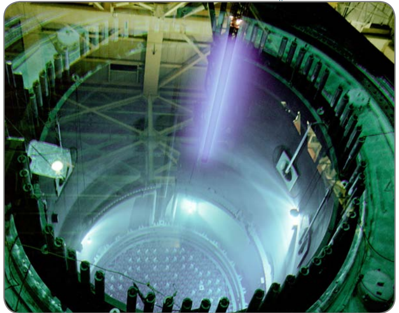
Nuclear fuel rod movement at Columbia Generating Station
