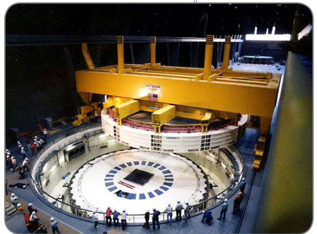
Stator units at Grand Coulee Dam Third Powerplant
