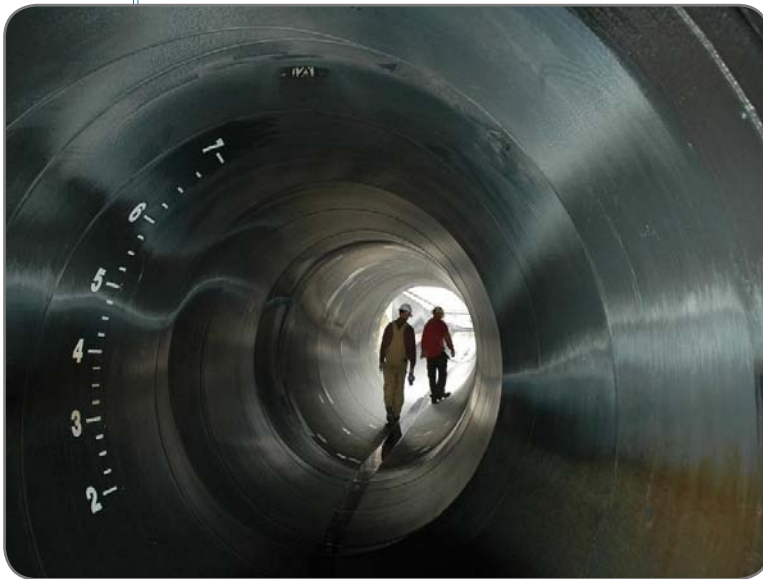
PUD employees take a maintenance walk through the juvenile fish bypass at Rocky Reach Dam
