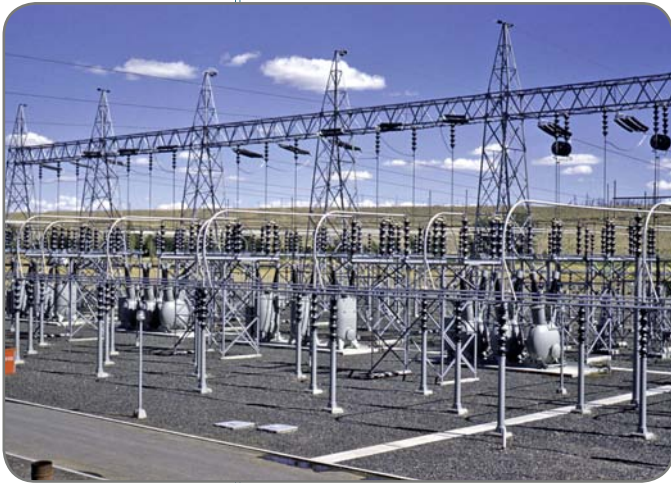
McNary Substation in Umatilla Oregon
