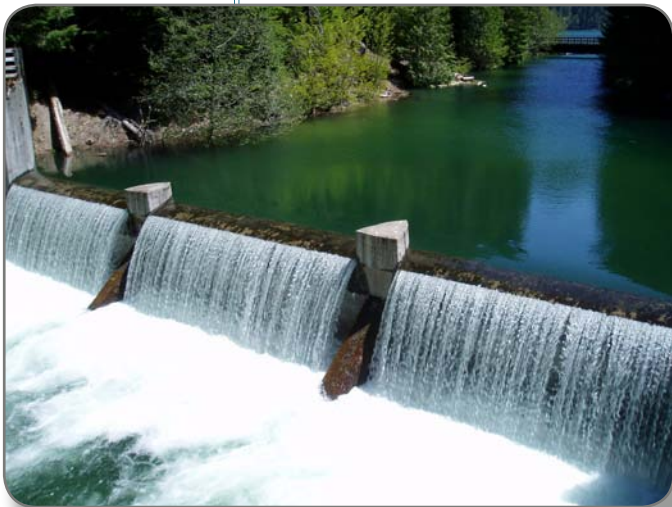
Overtopping at Packwood Lake Dam
