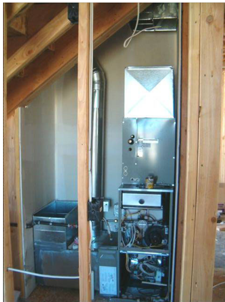
Figure 5. New Tradition Homes – Air Handler in Conditioned Space, under Stairwell
