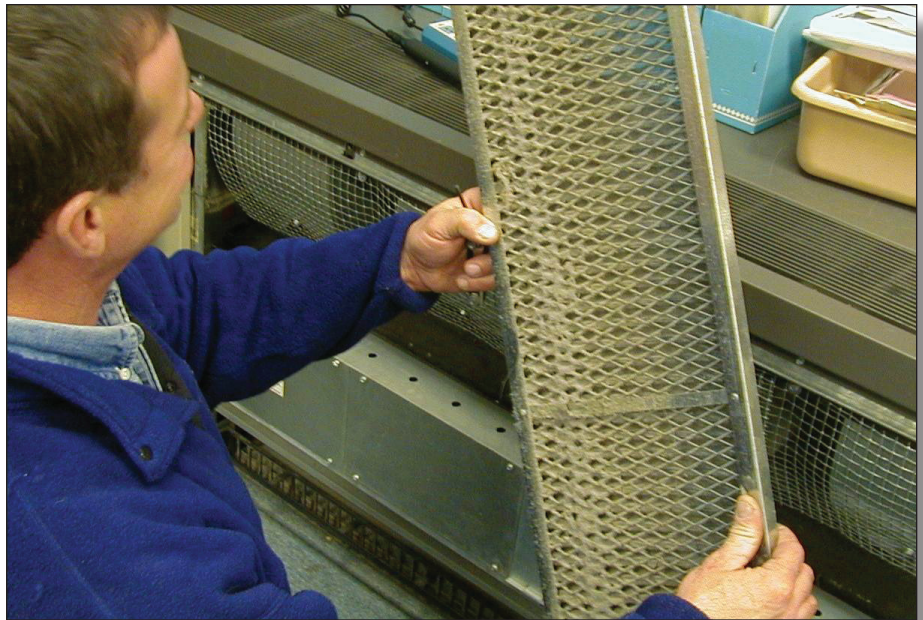
Make sure air filters are not clogged so the ventilation system can work properly. Photo: Rich Prill
