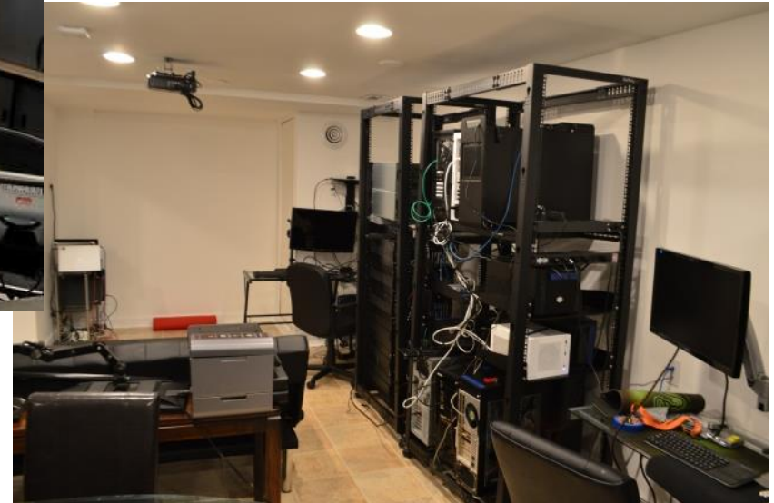
Server Rooms Served by Central HVAC
