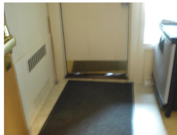
Gaps under doorways
