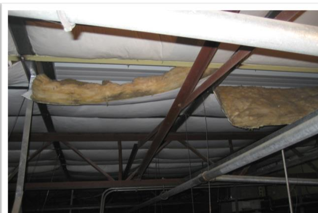
Failed roof insulation
