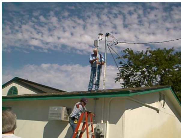
Figure 3: Weather monitoring system installation – Boise portable classroom
