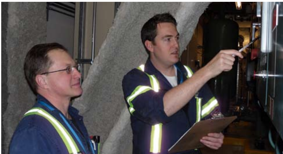
Kostyantyn Dubetsky (left) and Greg MacKintosh, power engineers with the Vancouver Convention Centre, survey the status of a 1500 ton York chiller/heat pump that uses seawater from Coal Harbour in heating and cooling.
