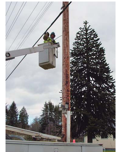
Utilities work to restore power to one of hundreds of downed power-lines in the Hoquiam/Grays Harbor area.
