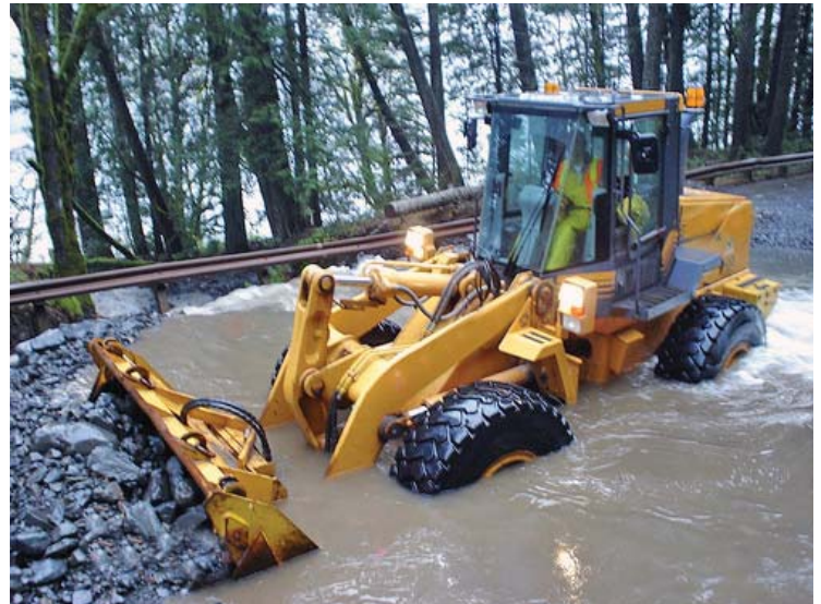
Washington Department of Transportation and many other Consortium members assisted in mitigating extensive flood damage in western Washington in December. Photo courtesy of WSDOT.
