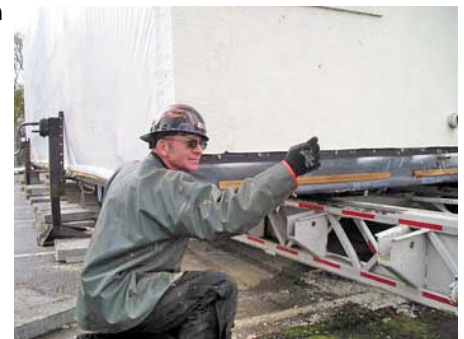
Jack Anderson, president of Interstate Modular, Inc., directs the movement of modular buildings on the state Capitol Campus.
