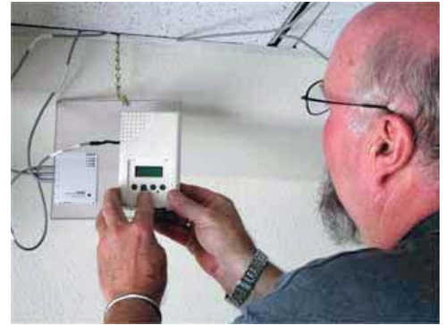
Keithly Barber Associates perform building diagnostic services on existing building systems to help determine the cause of any number of system issues.
