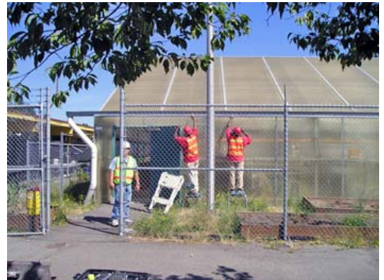
DOC staff begin the eight-day deconstruction process on the 40 x 70 sf greenhouse.
