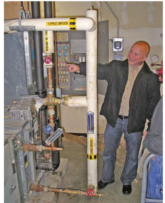
Jeff Vrabel, facilities manager for the City of Tumwater, leads the Consortium energy assessment team through Tumwater's City Hall building.
