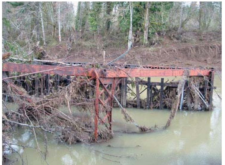
The gnarled metal remains of two bridges that were most affected by the Chehalis River floods have sunk into more than 12 feet of river muck, about 500 yards downstream from their original location.
