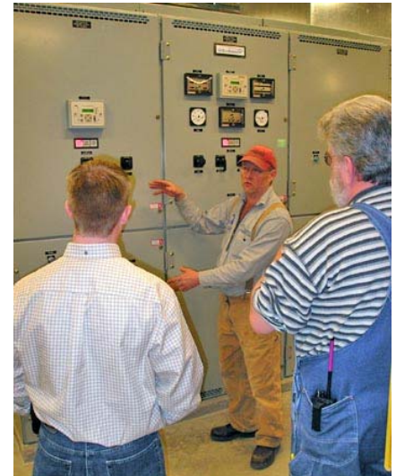
Bob Harding explains the complexities of Rainier School's new power grid.
