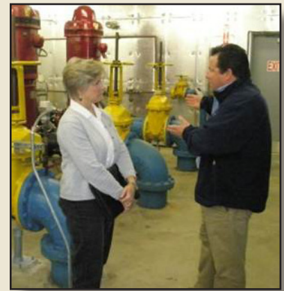
Deke Jones with Auburn City staff at Auburn water pumping station.
