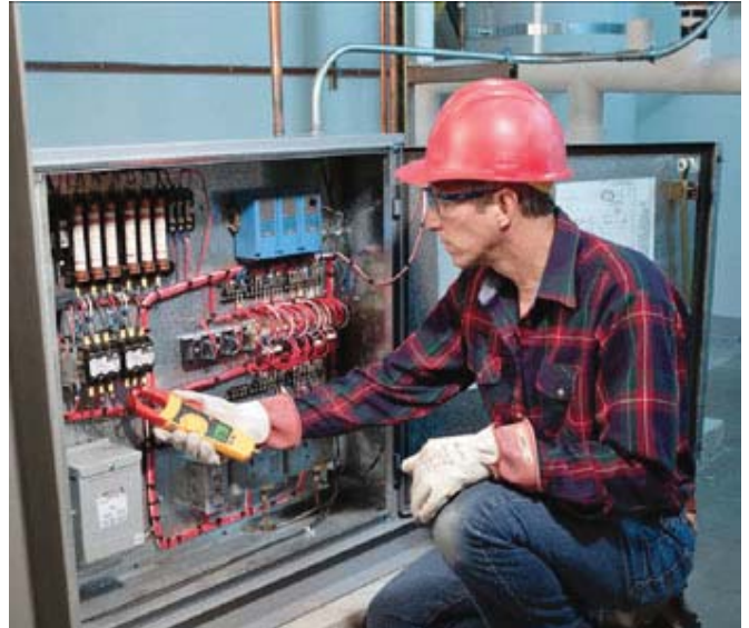
Figure 4 - Checking running current on the compressor controls.
