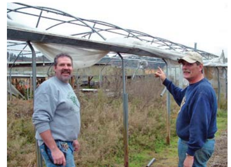
David Woody (l) and Greg Banner explain how their crew will disassemble one of the Kent greenhouses. The two Olympic Corrections Center members supervised a five-person crew during the deconstruction and transport of the systems.
