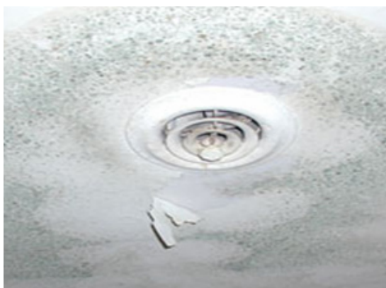
Mold surrounding air conditioning vent in ceiling due to water leak. (EPA photo, John Martyny, Ph.D.)
